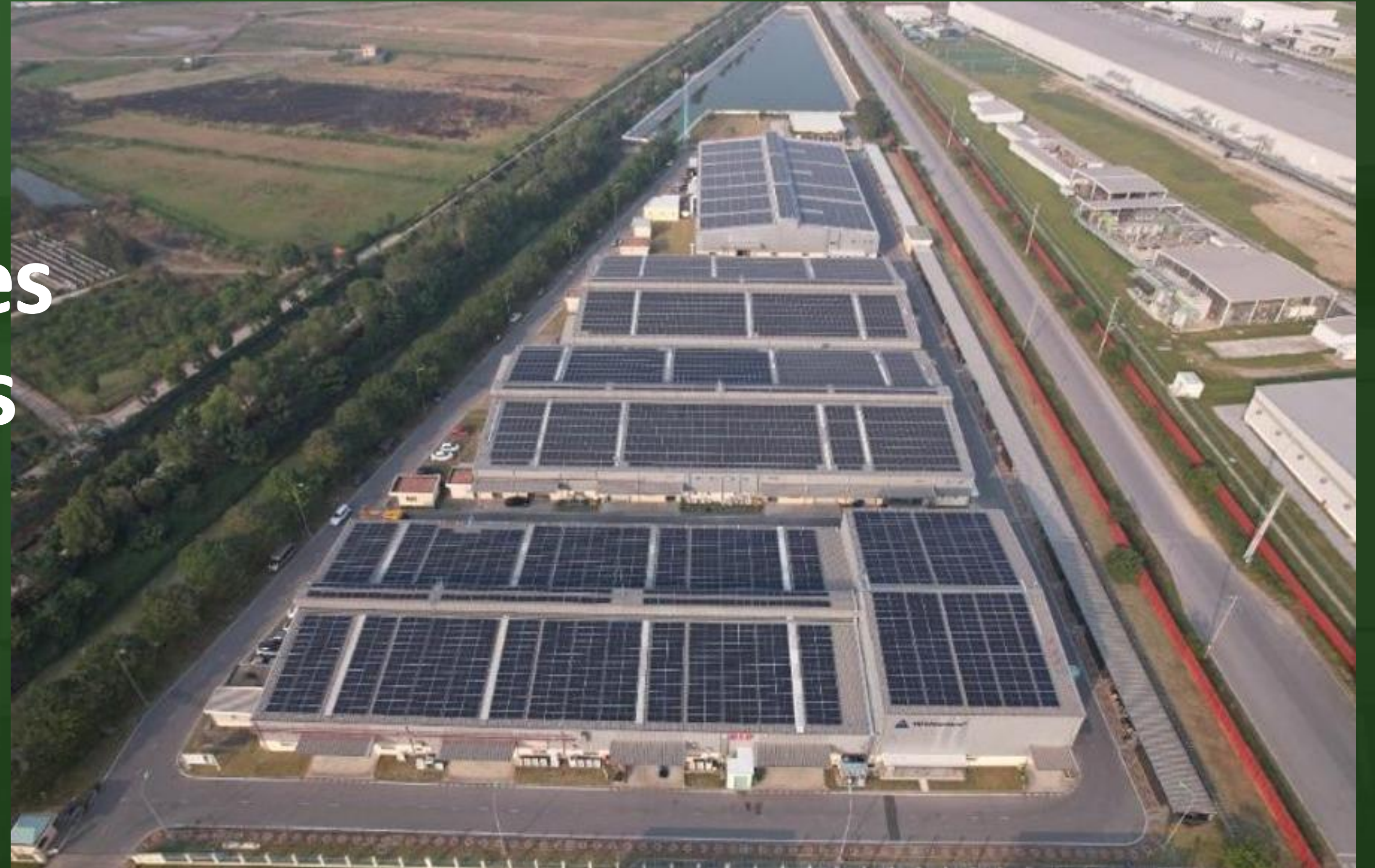
Rooftop Solar Project in Thang Long II Industrial Park Management Board
